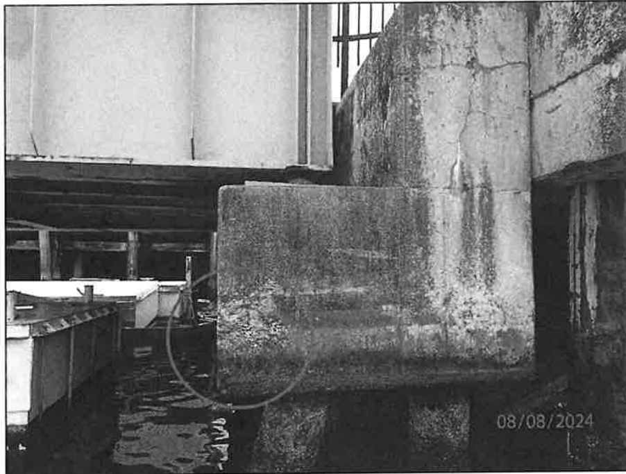
Photo 13 – Abutment North End (note spall)
