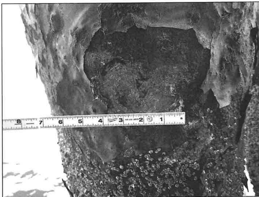
Photo 11 – View of up to 1/4" deep Section Loss at Hoist Tower Pile
