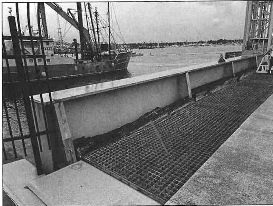
Photo 15 – View of Severe Rot and Section Loss of Timber Curb
