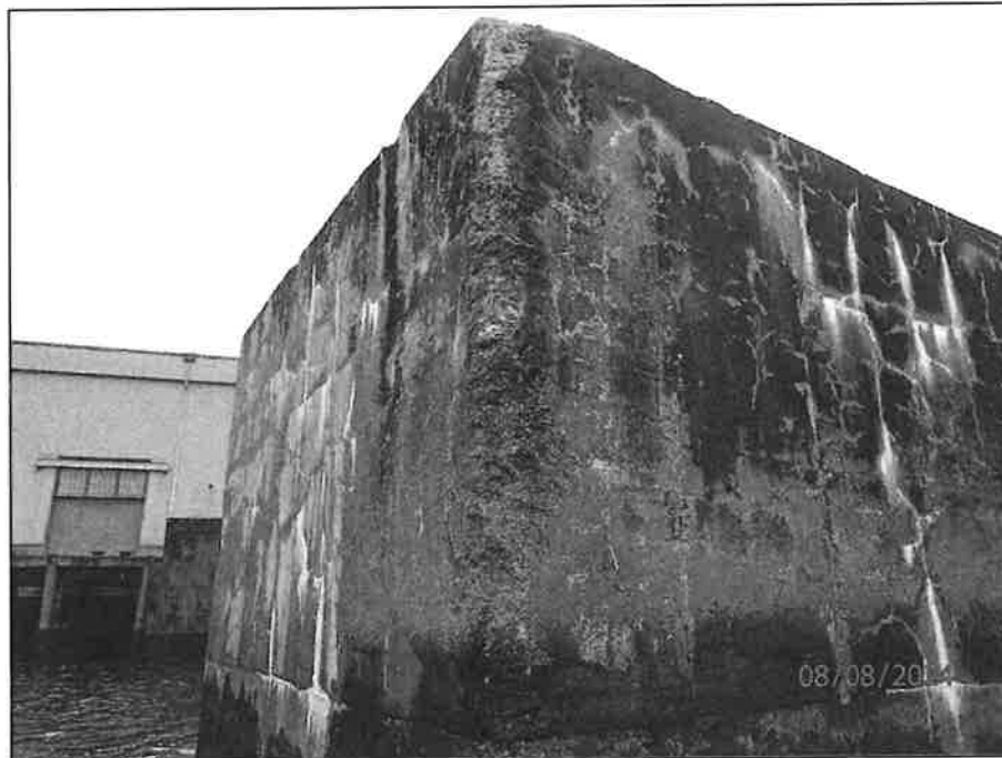
Photo 6 –Northeast Fender Dolphin scale/spall at northeast corner
