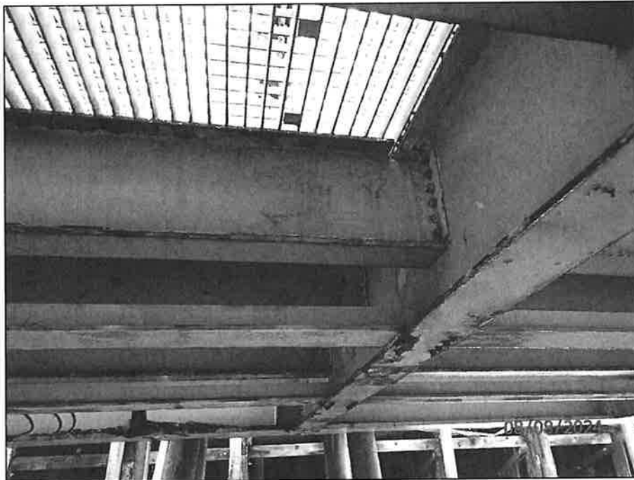
Photo 9 – Typical Missing/Peeling Paint and Corrosion of Ramp
