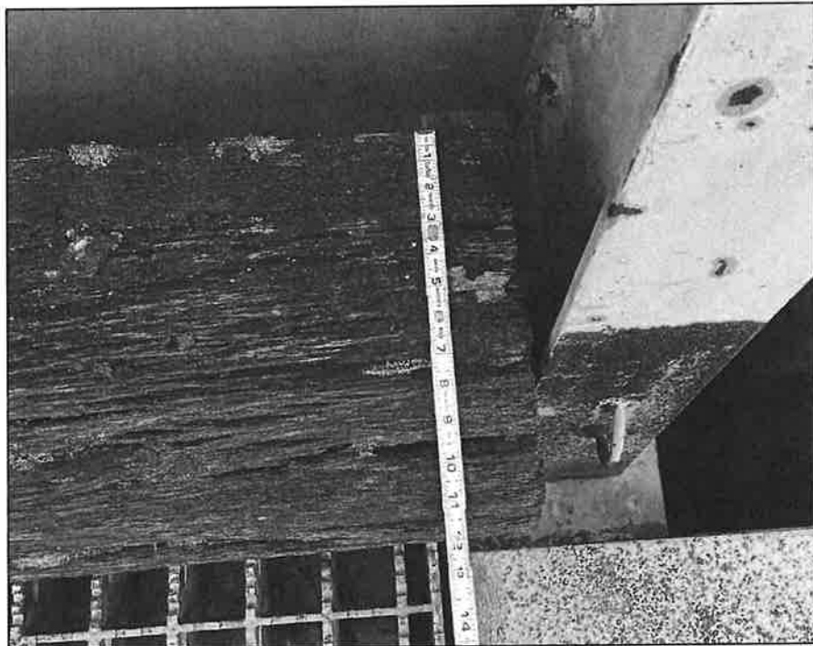
Photo 16 – Typical Timber Curb Condition
